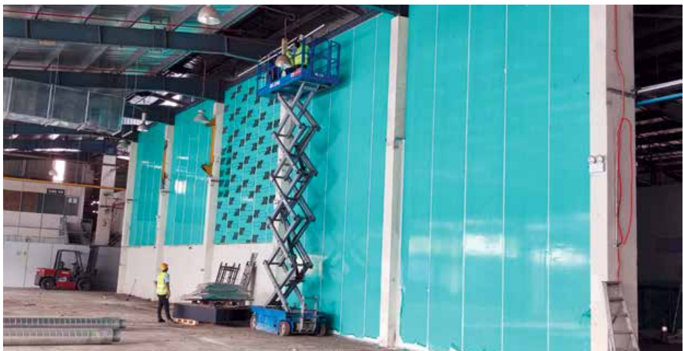
Super combi dry and solventless laminating line’s room partitioning work progress in September 2022.
